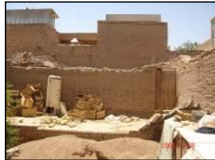
Figure 8. Devastated buildings in old city of Yazd Source: authors
