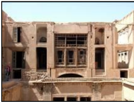
Figure 7. Devastated buildings in old city of Yazd Source: authors
